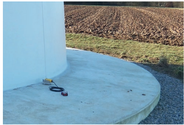
Figure 4.8-1: Vibration measurement point MP A at the tower foundation of WT 5. Photo: Wölfel company
